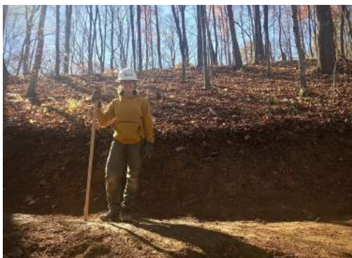
Lillian Cahill, Appalachian Conservation Corps crew member, constructing the Baileys Trail System, November 2020.
